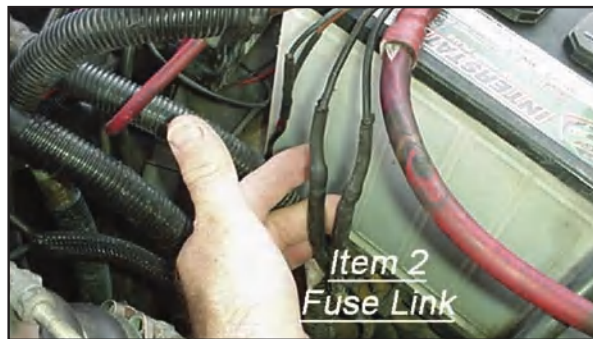
Also check the fuseable link that feeds the solenoid (Item 2) or fuse #9 in the fuse panel.
