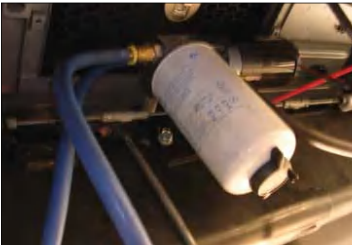
The FASS unit from the underside.
