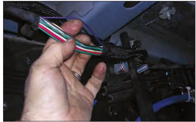
Intercept the wiring harness at the area of the driver's door and you can manually operate the fuel transfer pump.
